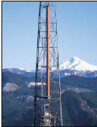
KWOP Channel 33/31, Salem, Oregon The site-mounted, dual adjacent, TRASAR antenna operates both NTSC & DTV signals simultaneously.
